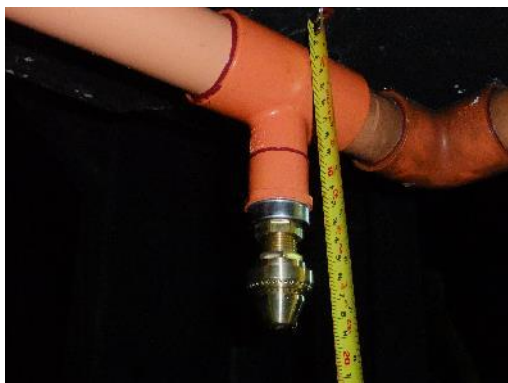
Ceiling mounted pipe and nozzle
